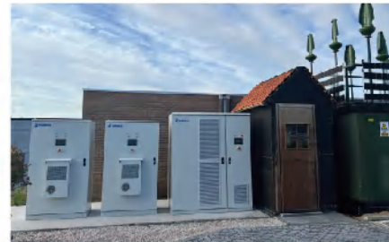
Hotel, Belgium Capacity: 250kW / 430kWh Application: Demand Response
