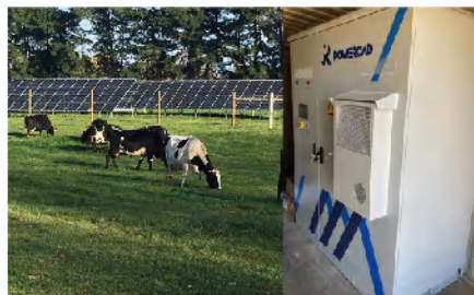
Dairy Farm, New Zealand Capacity: 60kW / 122.88kWh Application: Off-grid, Solar Self-consumption
