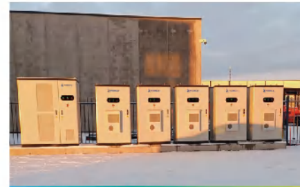
Equipment Rental Company, Norway Capacity: 500kW / 1075kWh Application: Peak Shaving, Balancing Services
