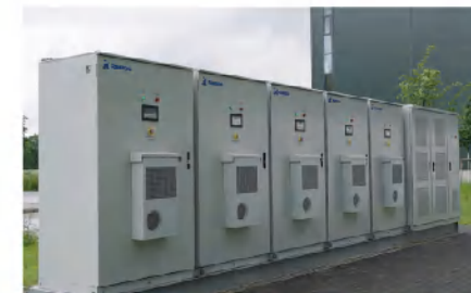
Distribution Center, Germany Capacity: 500kW / 1000kWh Application: Solar Self-consumption
