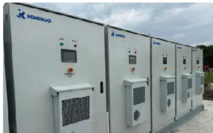
Pig Farm, Netherlands Capacity: 1.5MW / 3MWh Application: Balancing Services
