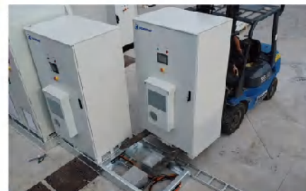
Chicken Farm, Belgium Capacity: 250kW / 430kWh Application: Balancing Services
