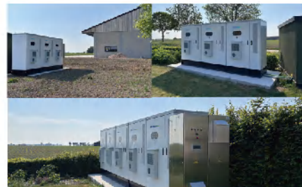
Quinoa Farm, Belgium Capacity: 1.1MW / 2.3MWh Application: Solar Self-consumption, Balancing Services
