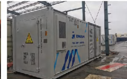
Electrical Equipment Factory, Mexico Capacity: 187.5kW / 648kWh Application: Solar Self-consumption
