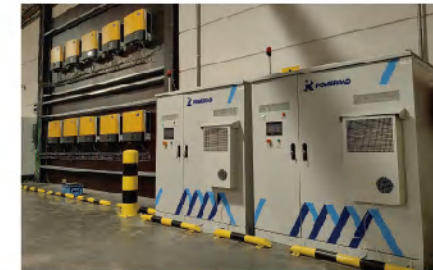
Chocolate Factory, Belgium Capacity: 350kW / 748kWh Application: Backup Power
