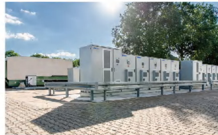
Logistic Fleet Charging Station, Netherlands Capacity: 1.5MW / 3.2MWh Application: Solar Self-consumption, Balancing Services
