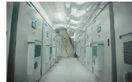
Stadium, Netherlands Capacity: 2MW / 5.59MWh Application: Peak Shaving
