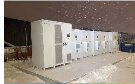
EV Charging Station, Sweden Capacity: 500kW / 1075kWh Application: Balancing Services
