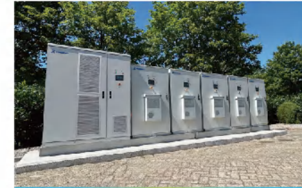
Glass Factory, Netherlands Capacity: 500kW / 1000kWh Application: Solar Self-consumption
