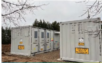
PV Panel Factory, Lithuania Capacity: 1000kW / 2580kWh Application: Solar self-consumption, Peak Shaving
