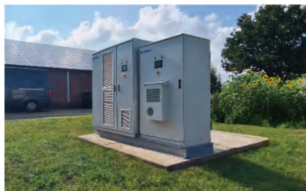
Livestock Farm, Netherlands Capacity: 62.5kW / 215kWh Application: Solar self-consumption, Balancing Service
