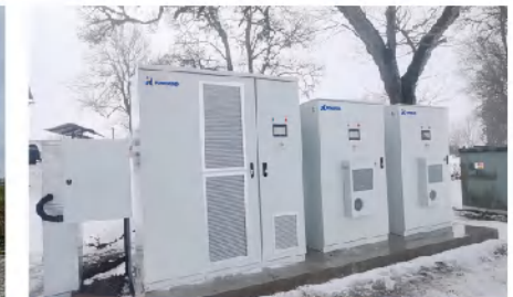
Sweden Capacity: 187.5kW / 430kWh Application: Frequency Regulation
