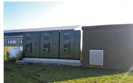
Chicken Farm, Belgium Capacity: 300kW / 645kWh Application: Solar self-consumption, Balancing Services
