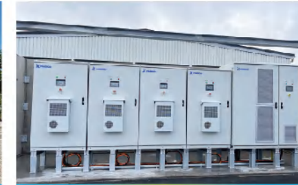
Steel Processing Factory, Sweden Capacity: 500kW / 860kWh Application: Frequency Regulation
